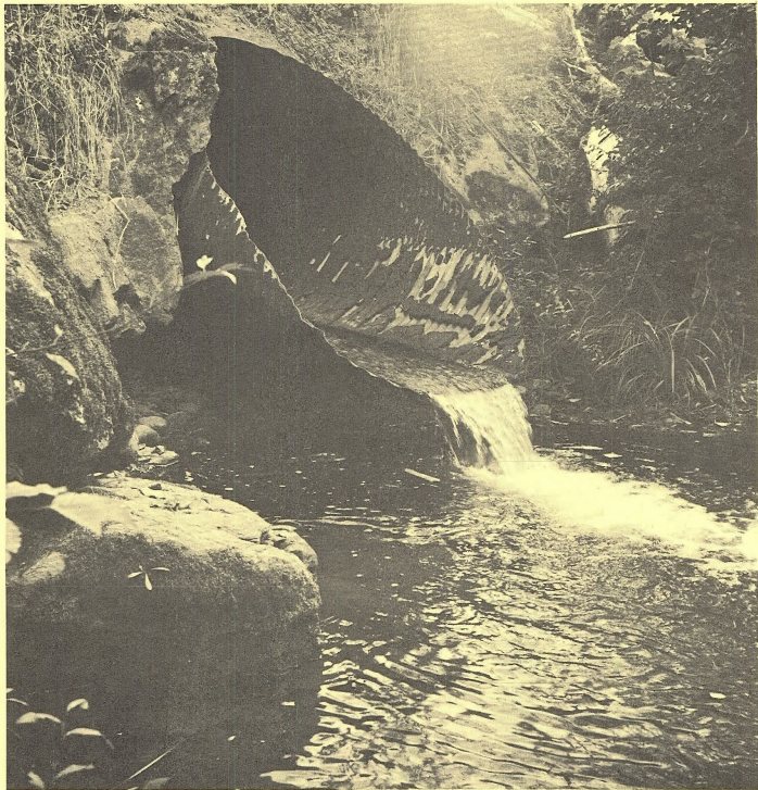
Illustration 3 - GOLD CREEK - Culvert outlet before dams were built. Overhang prevented passage of salmon and steelhead.
